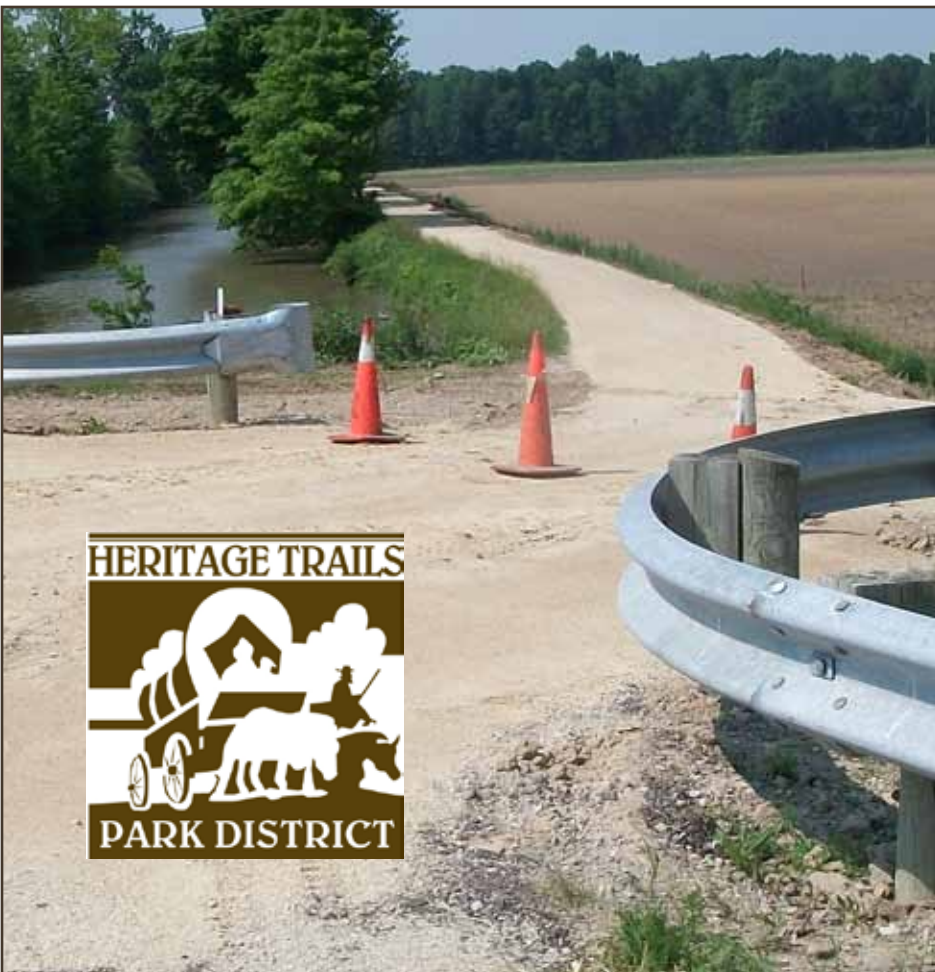
Improved section of the Towpath Trail where it intersects with St. Rt. 66 between Spencerville and St. Marys.
